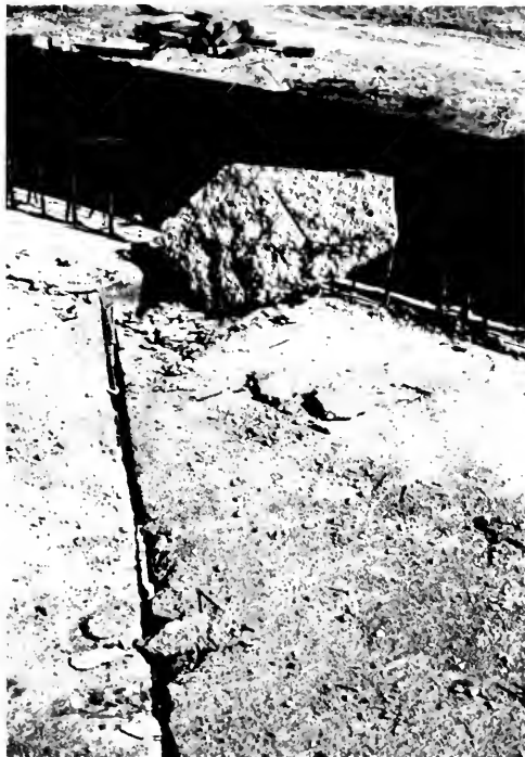
Photo 29. Pounding damage at expansion joint, Santa Clara overhead crossing on State Highway 14.
